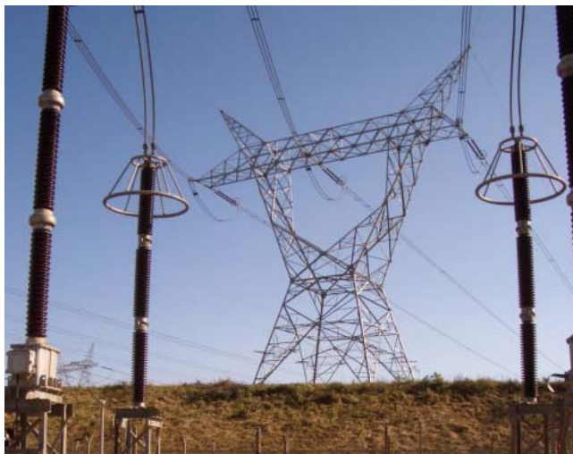
FIGURE 8 – First tower of the 22 km - 400 kV line
