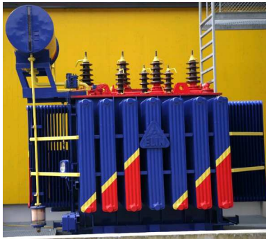
Figure 2: 6,5 MVA, 47 kV/27,2 kV power transformer
