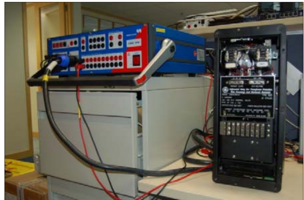
Figure 1: Test setup for testing EM relay (Transformer differential relay BDD from GE)
