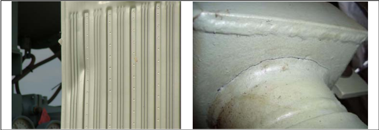
Figure 10: Bumping marks indicating possible damage of this transformer after its shipment
