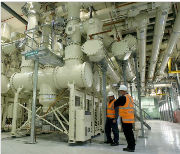
Figure 1: Example GIS Turnkey Indoor Substation
