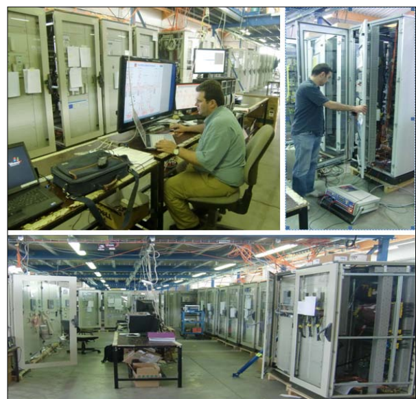
Figure 3: Factory test: control system (a.l.), protection panel test (a.r.), control-protection-metering interconnection (below)
