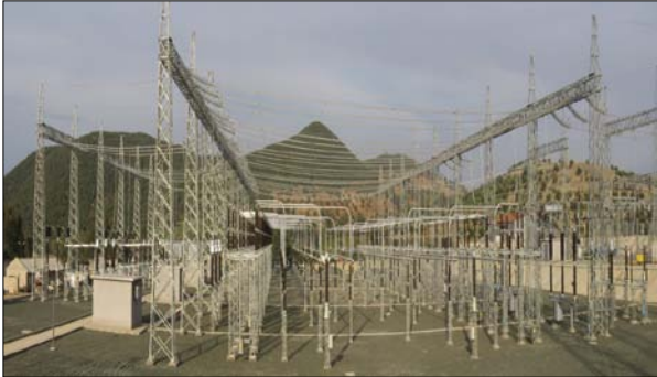
Figure 9: 400 kV AIS Substation "OPTI" (name changed)
