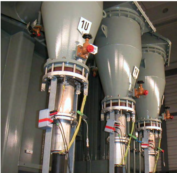
Fig. 24: 110 kV transformer inlet
